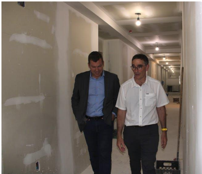
Polycorp Group of Companies owner Peter Polley, right, takes Kings-Hants MP Kody Blois on a tour of the new apartment building under construction at Woodman’s Grove in Wolfville. It will include 72 suites with 60 of them being affordable housing units. - Jason Malloy
